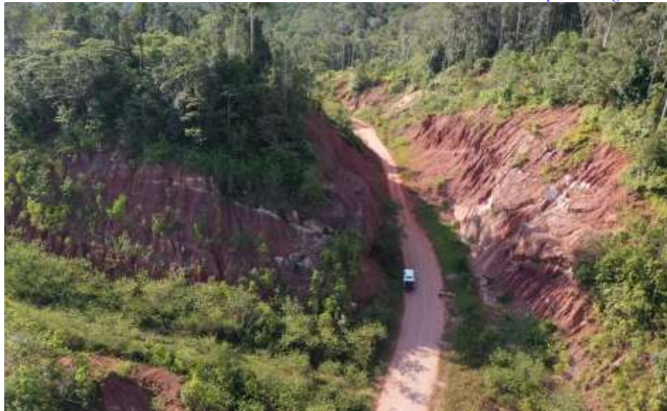
Figure 1. Photography of Slope in Km. 234+600 Road Section of Sisu – Snopy Papua Barat Province
