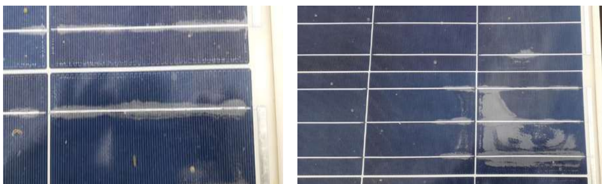
Figure 2. Hsl250 Defective Solar Panels From Hanhwa.
