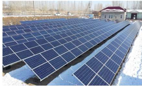
b) General View of Namangan-Pop Solar Photovoltaic Power Plant
