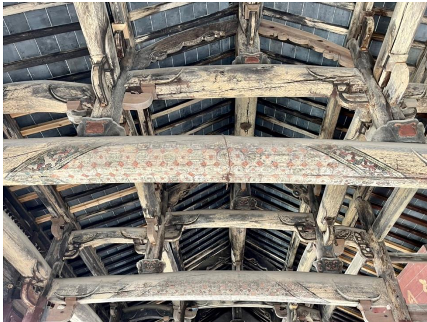
Figure 2. Baofujin Color Painting Decoration of Wooden Beams in The Interior of The Gaoyang Bridge
